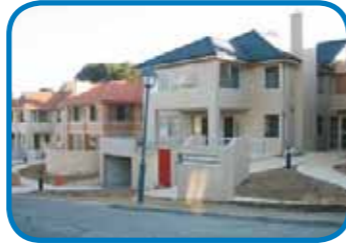
The first two blocks are occupied and will soon begin to take shape on the outside.
